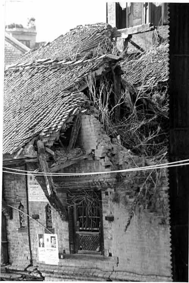
Collapsed roof structure at southeast corner of the building.
